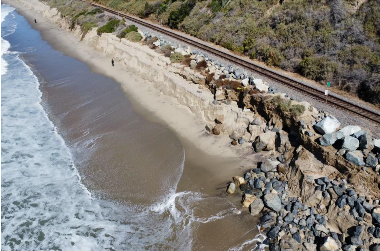
Figure 33. Aerial View of Little to No Shore Protection South of San Clemente State Beach Near MP 206.6
