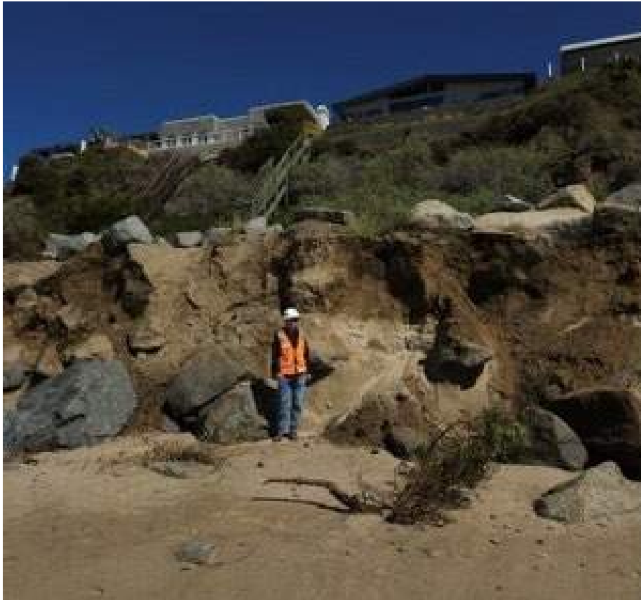
Figure 17. Potential Reinforcement Site 4: MP 206.00 to 206.67, North End of Cyprus Shore Project, July 2023
