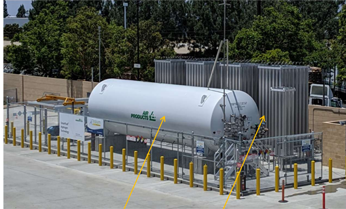
Liquid Storage Tanks and Vaporizers - Leased
