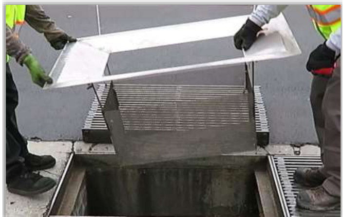
Grated Inlet Trash Screen
