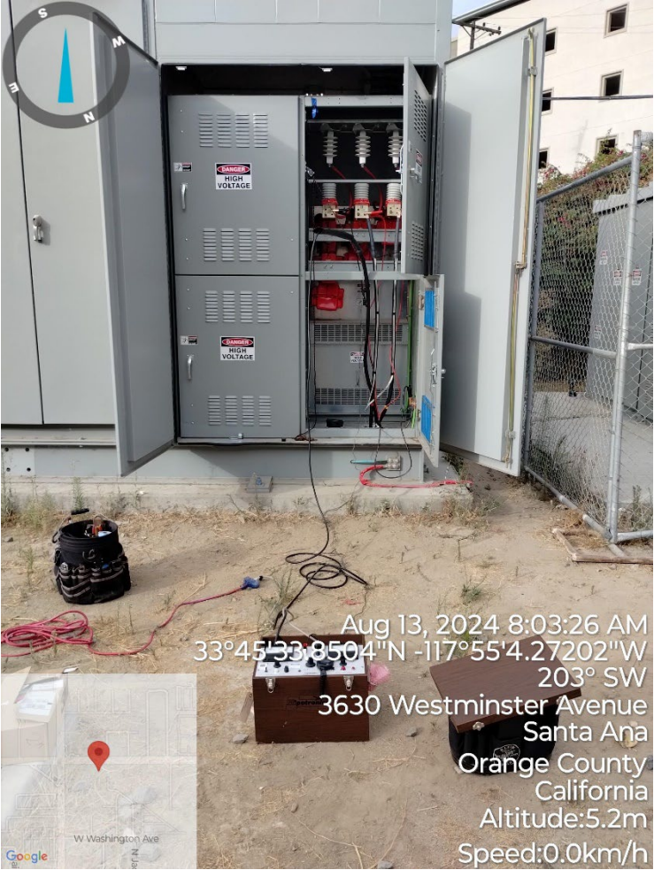
Traction power substation No. 1
