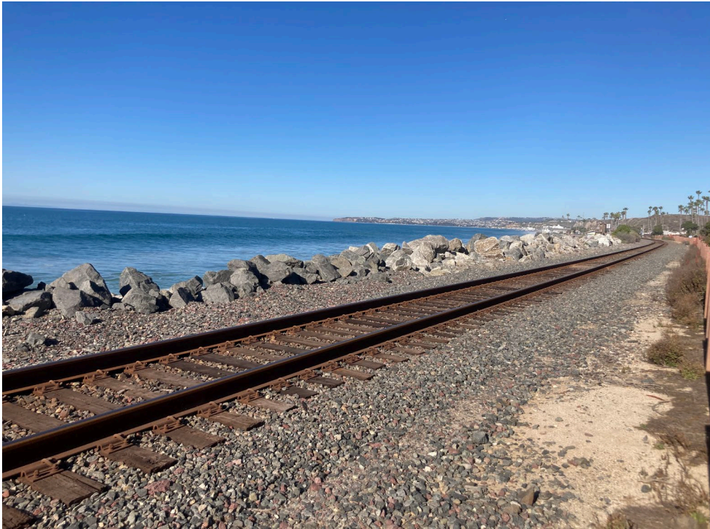
MP 203.80 - 203.90: Erosion Hazard deteriorating
