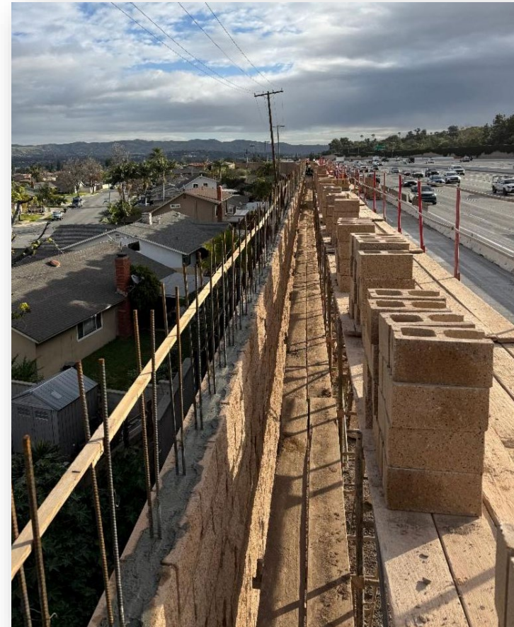
Preparation for placing blocks that form the top of the sound wall along the westbound SR-91 on-ramp
