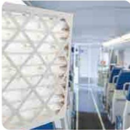
Antimicrobial air filters in train ventilation system
