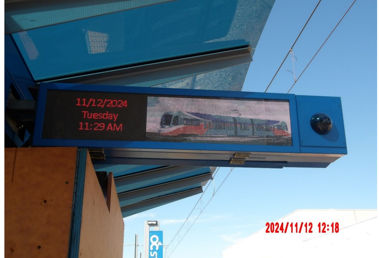
Variable Message Sign at Fairview Platform
