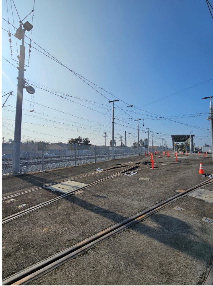
Installed OCS Wire and Fence
