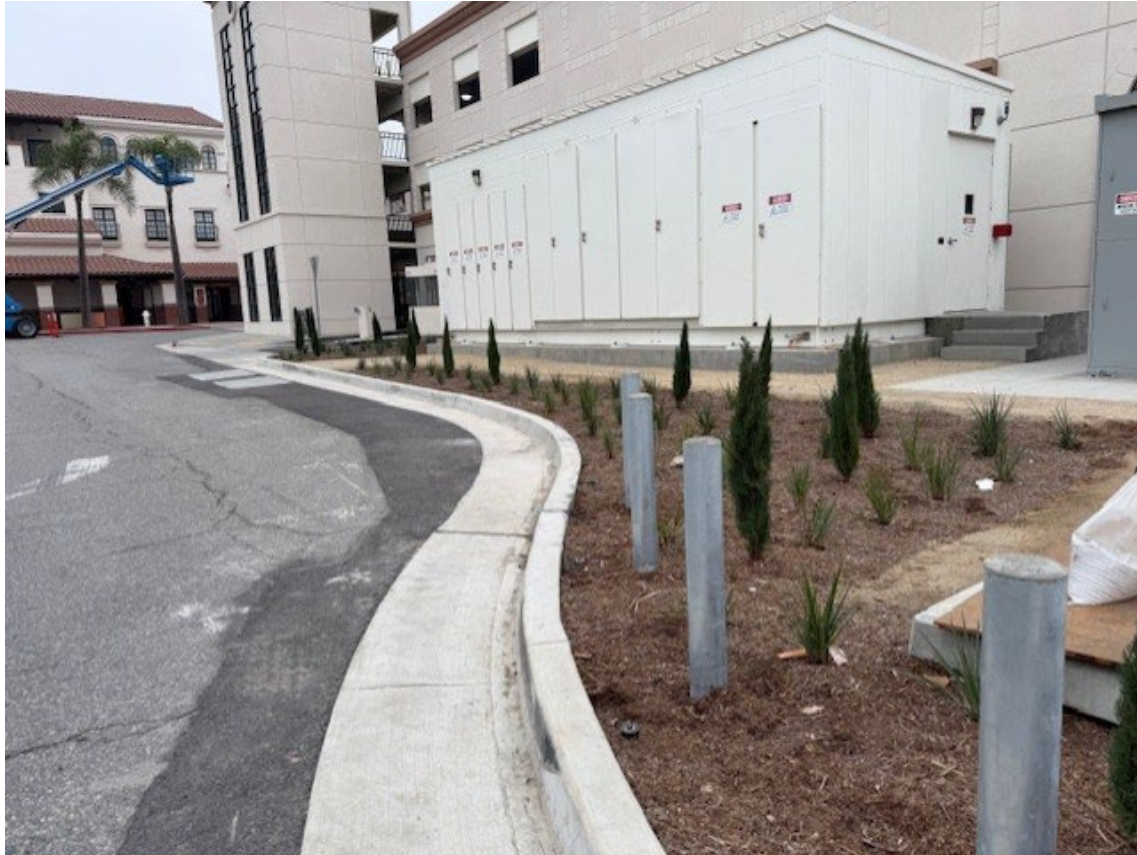
Traction Power Substation 4
