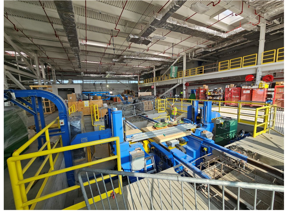
Interior of MSF
