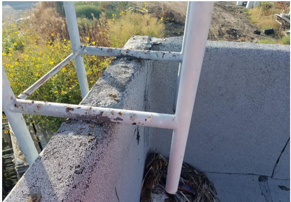
Photograph 10: View of bird droppings at exterior roof access ladder.
