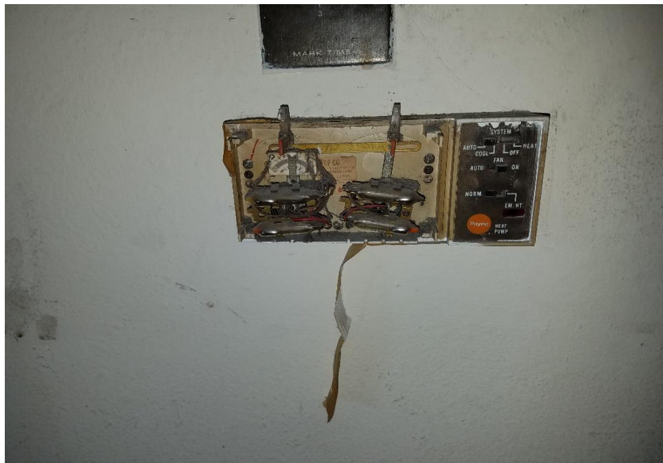
Photograph 12: View of representative mercury-containing thermostat switches.
