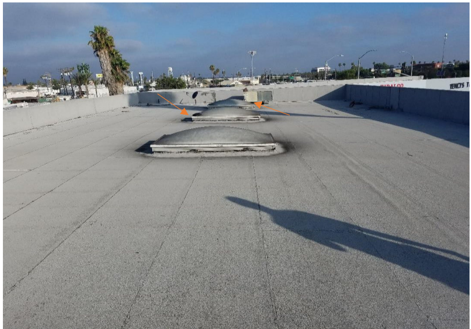
Photograph 2: View of the asbestos containing penetration mastic and HVAC seam mastic.
