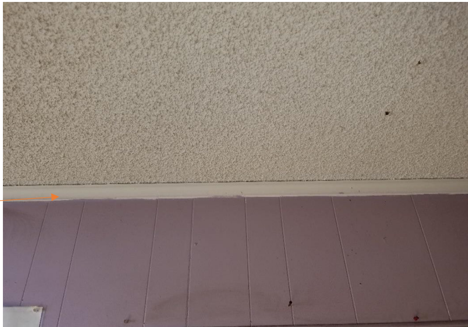
Photograph 8: View of the lead-containing white wood crown molding in Unit 1516 office and break room.
