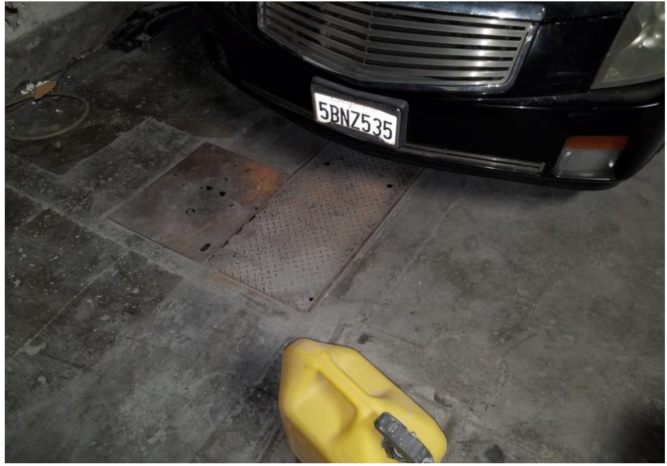
Photograph 15: View of either oil pit or clarifier located in Unit 1514.
