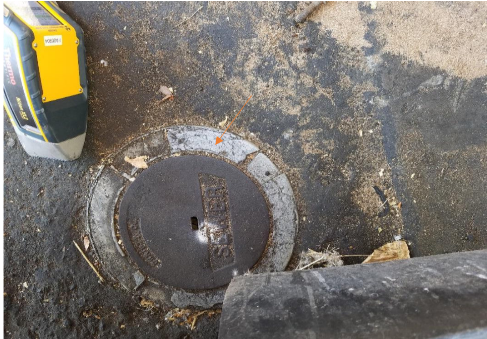
Photograph 6: View of the lead-containing paint sewer grate in a poor condition.
