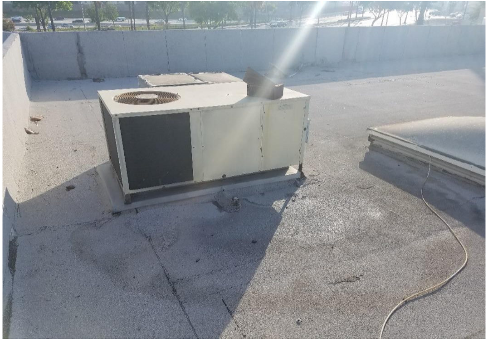
Photograph 9: View of exterior rooftop HVAC units.
