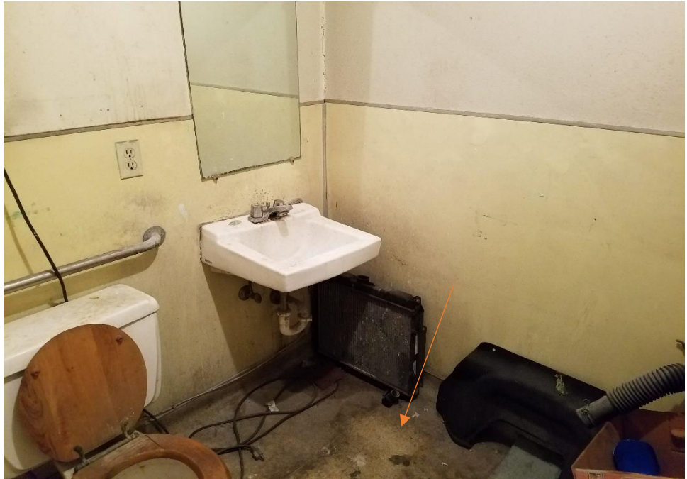
Photograph 3: View of the asbestos containing vinyl floor sheeting in Unit 1518 restroom.
