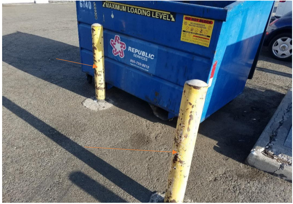
Photograph 5: View of the lead-containing paint on bollards with paint in a poor condition.
