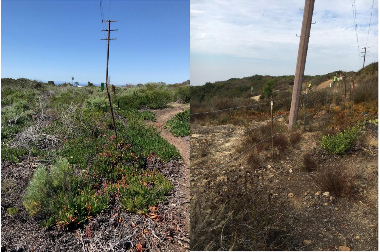
(Left) Old rusty barbed wire fence line. (Right) New smooth wire fence line (wildlife friendly). Contractor was able to utilize some of the same posts. Fence is in the same location.
