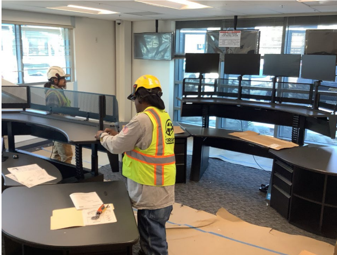
Operations Control Center
