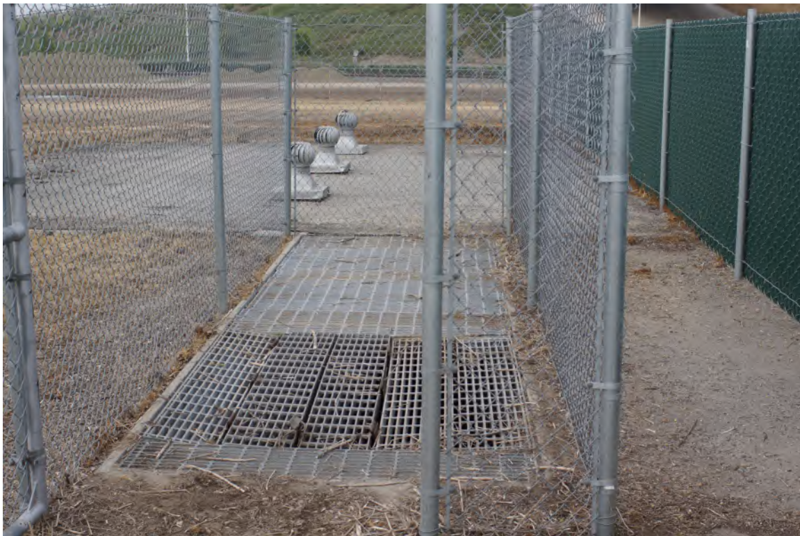
Figure 3.3.5-3 Overview of Water Transfer Vault from surface, View to West
