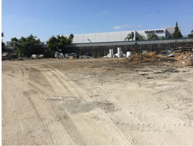
Photograph 14. View of storage on the southern portion of the site, behind the locked gate, facing south.
