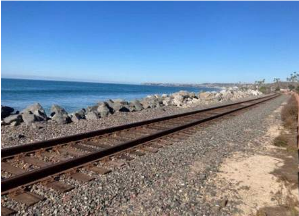
Figure 12. Potential Reinforcement Area 1: MP 203.85, November 2023
