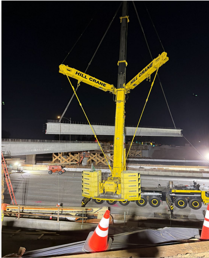
Placement of girders, steel beams, which will form the structural backbone of the Lakeview Avenue bridge
